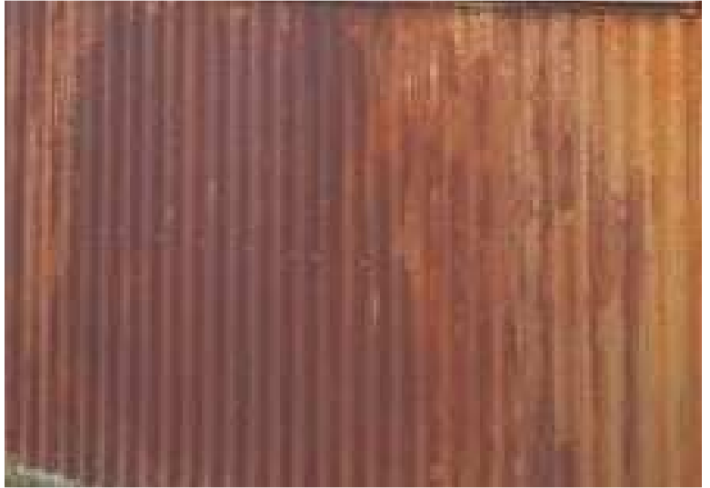
I - rusted corrugated metal siding
