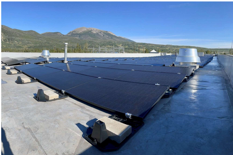
Public Works Solar Rooftop Solar
