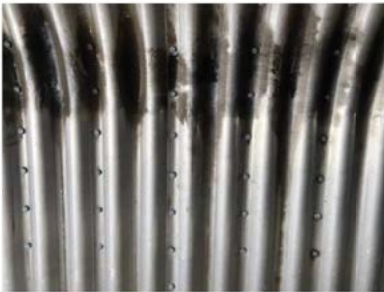
Close Up of the interior texture of the tunnel. See pgs 7 & 8* for concept.
