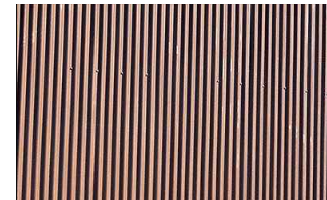
METAL SIDING: 7/8" CORRUGATED (RUSTED)
